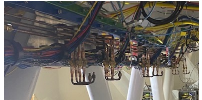
CO2 Piping in Test Cell TCS
